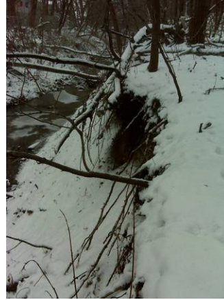
Figure 5. Photo taken at number 4 in Figure 1. Displays an erosion and undercutting severity of 3.
