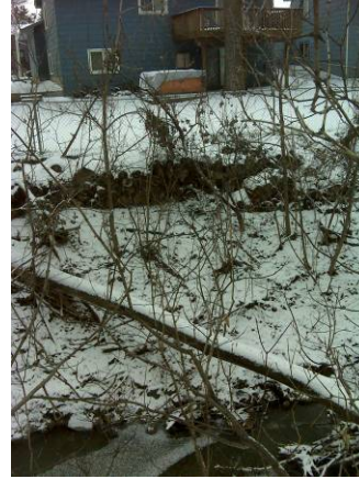
Figure 6. Photo taken at number 5 in Figure 1. Displays an erosion and undercutting severity of 3.
