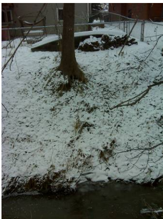
Figure 10. Photo taken at number 9 in Figure 1. Displays an erosion and undercutting severity of 3.
