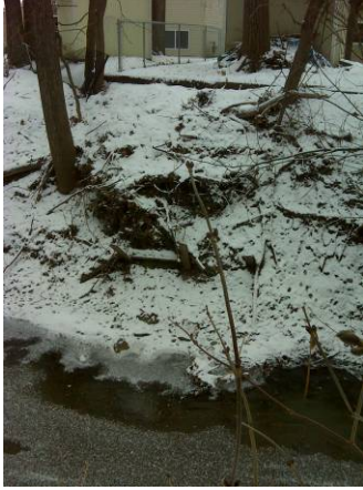
Figure 2. Photo taken at number 1 in Figure 1. Displays an erosion and undercutting severity of 3.
