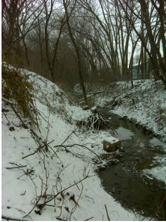
Figure 8. Photo taken at number 7 in Figure 1. Displays an erosion and undercutting severity of 3.
