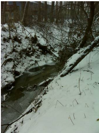
Figure 4. Photo taken at number 3 in Figure 1. Displays an erosion and undercutting severity of 3.
