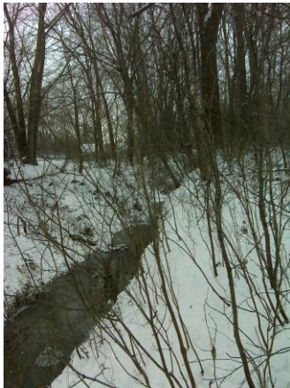
Figure 9. Photo taken at number 8 in Figure 1. Displays an erosion and undercutting severity of 3.
