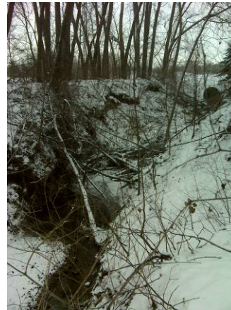
Figure 12. Photo taken at number 11 in Figure 1. Displays an erosion and undercutting severity of 3.
