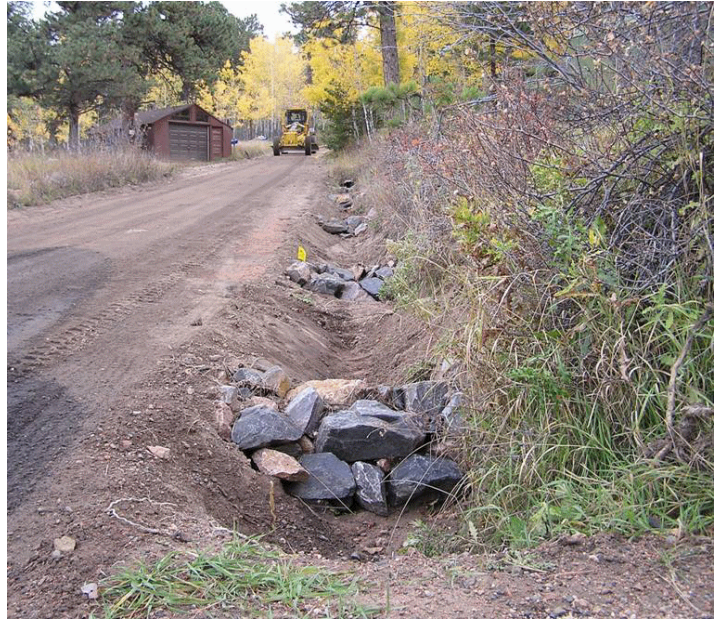
Figure 11: Rock check dams in a small ditch ( www.casfm.org/stormwater_committee/LID-Summary.htm )
