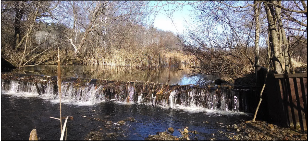
Figure 37 Deteriorating weir structure, November 2017
