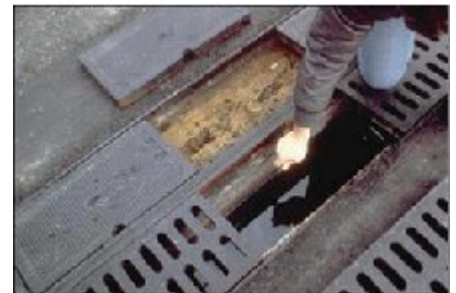
Typical sand filter. Source: Iowa Stormwater Partnership.
