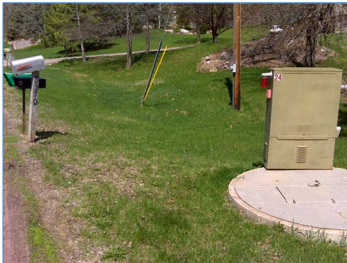
Figure 8: Sewage Pump Station
